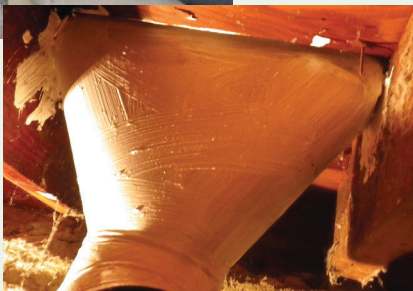
Right: Scraped and encapsulated boot (part of HVAC system).
